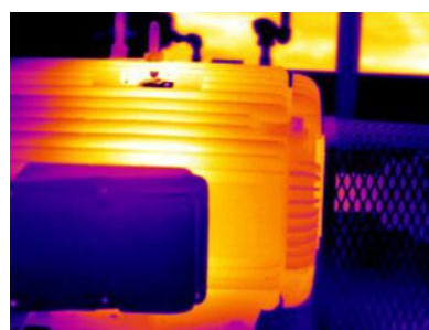
Infrared Imaging helps to spot potential problem and prevent downtime in mechanical systems
