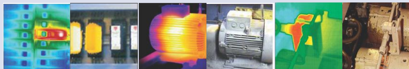
Electrical: Hot Fuses
